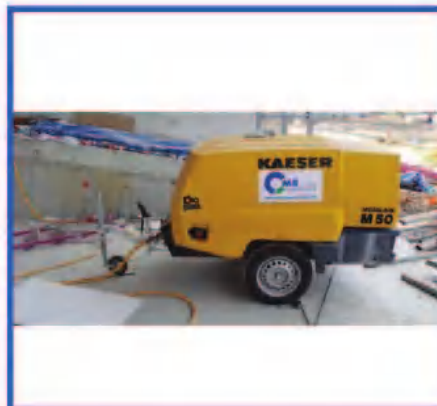
Air Compressor 2 units
